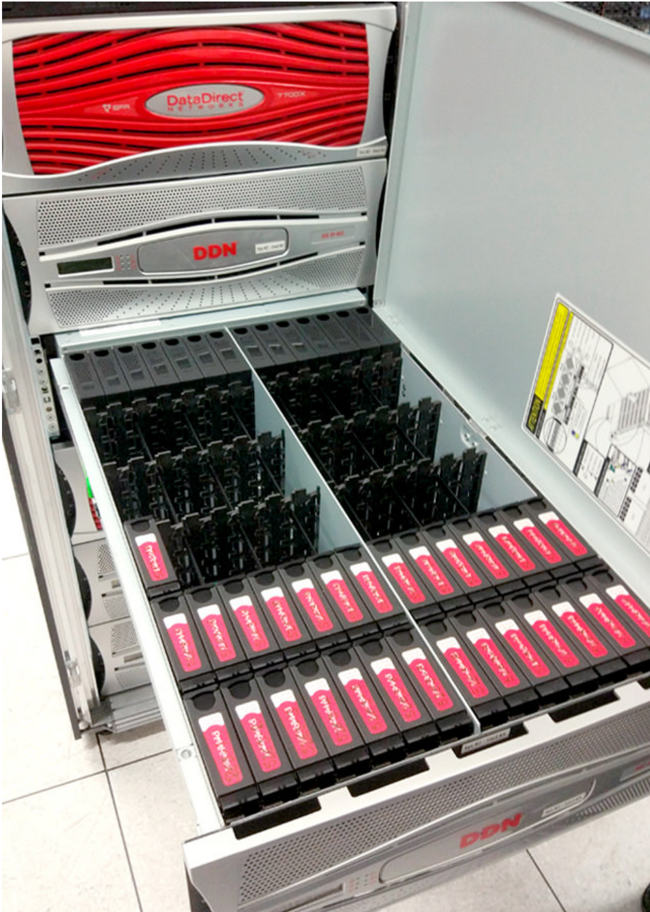
Barcelona Supercomputing Center
